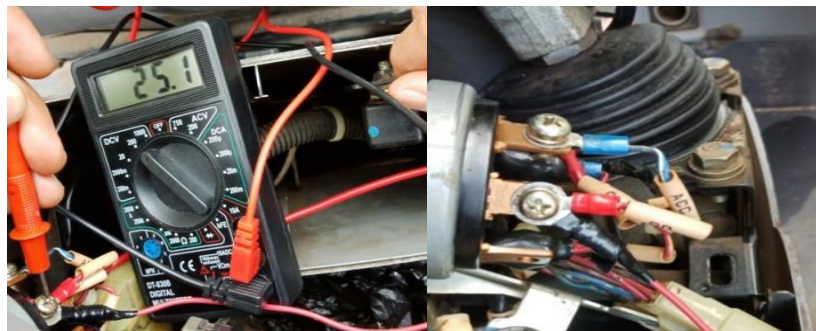
Figure 8: B+ Starting Switch Installation
