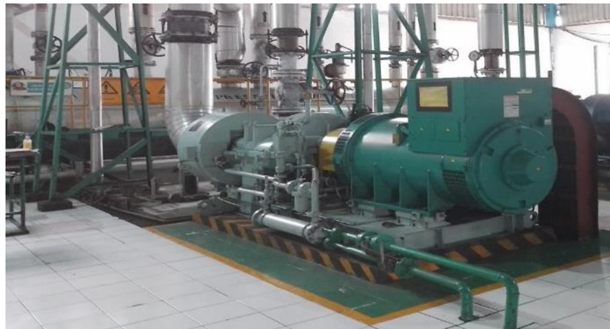
Gambar 1. Mesin turbin uap PT. KSA
