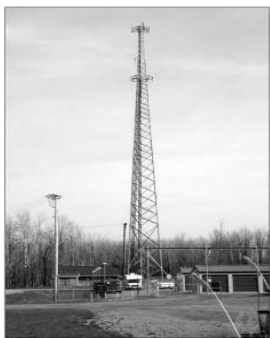
Gambar 4. Self - Supporting Tower
